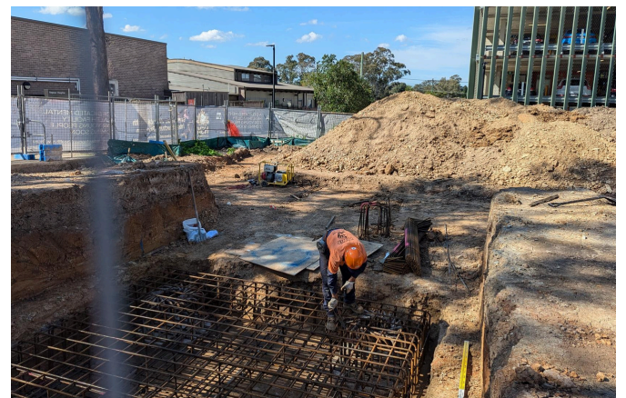
(Above) Piling works at the site of the new CAMHS Unit are complete
