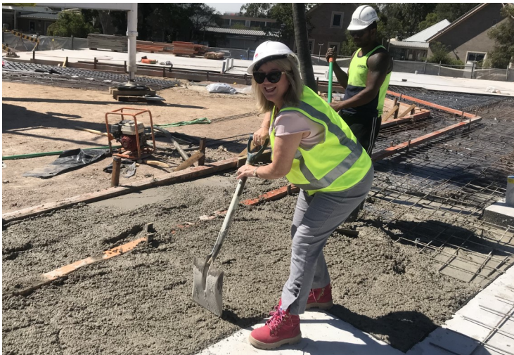
Nina Cleary from the redevelopment team at the final concrete pour for the childcare centre.
